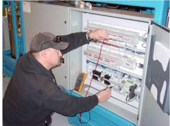
Jeff Halverson works on the electrical components on the skid headed for Europe.
