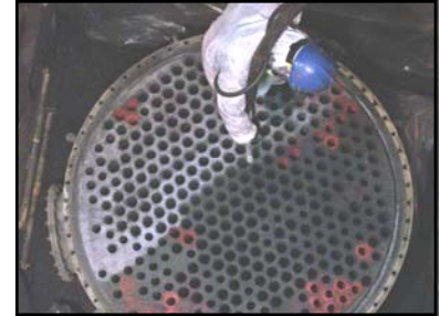
JD Atkinson stand on top of the heat exchanger unit. In the photo, the line of clean vs. dirty is clearly visible.
